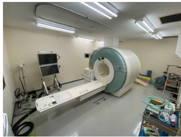
3T MRI scanner room
