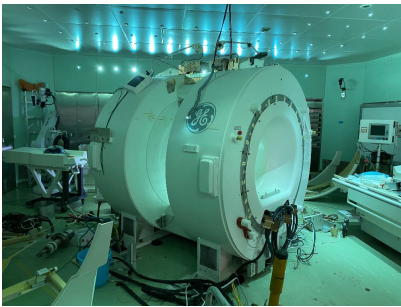
Interventional MRI room after quenching 2022, Shiga University of Medical Science Hospital
