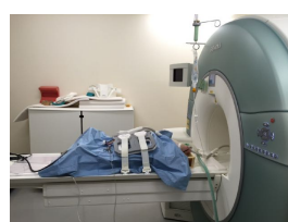
3T MRI scanner room
