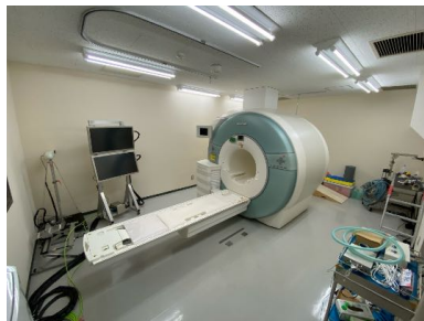
3T MRI scanner room
