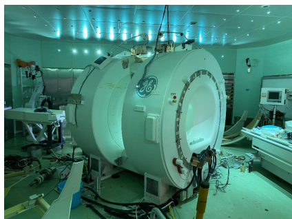
Interventional MRI room after quenching 2022, Shiga University of Medical Science Hospital
