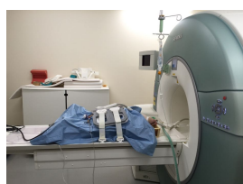
3T MRI scanner room
